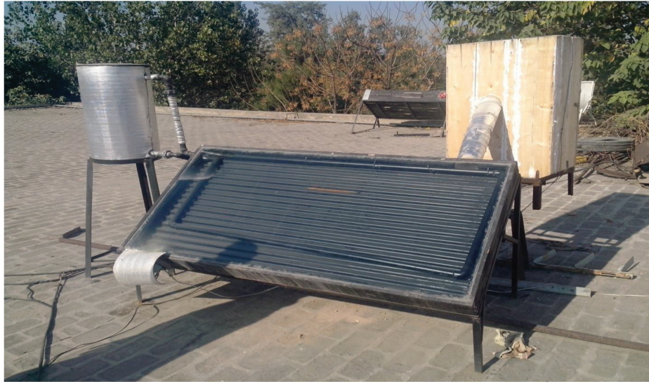
FIGURE 1. General view of the flat plate solar air heater
