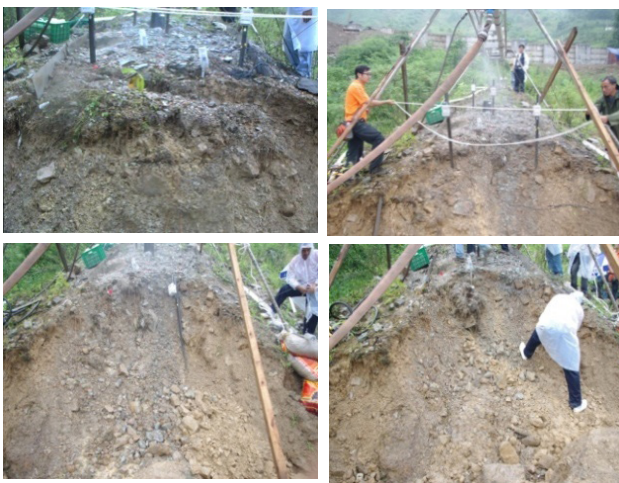
FIGURE 7. The final shape of scarp and slope failed progressively in the test
