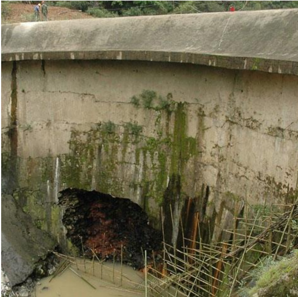
The damaged Boluokeng power station dam in Yingde City of southern China's Guangdong Province
